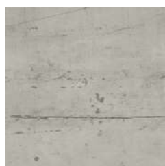
p40 Cold Cracked Concrete
